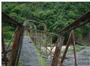
This is the broken foot bridge that villagers must cross to get to Kingston when hurricane season strikes. All photos by Nigel Male
